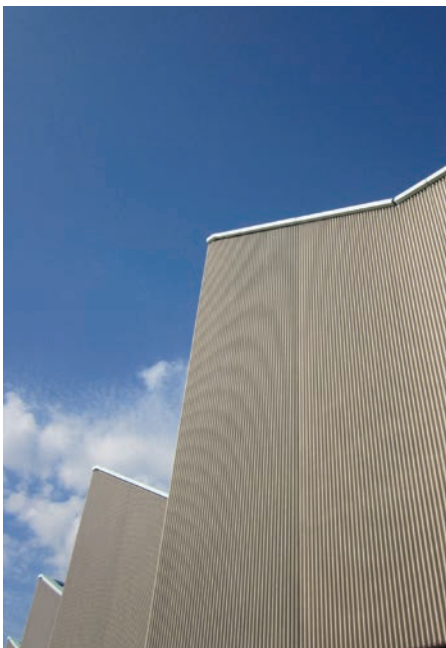
Specialism Building ribbed pre-cast concrete
