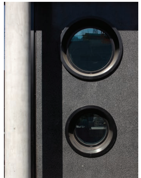
Podium wall punctuated by circular windows, which are framed with black power coated metal
